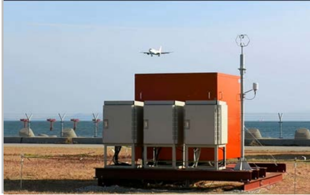
SOLWIN (Sodar-based Low-level Wind Information) 3-D Wind profile (HW, XW, Vertical) above Runway threshold
